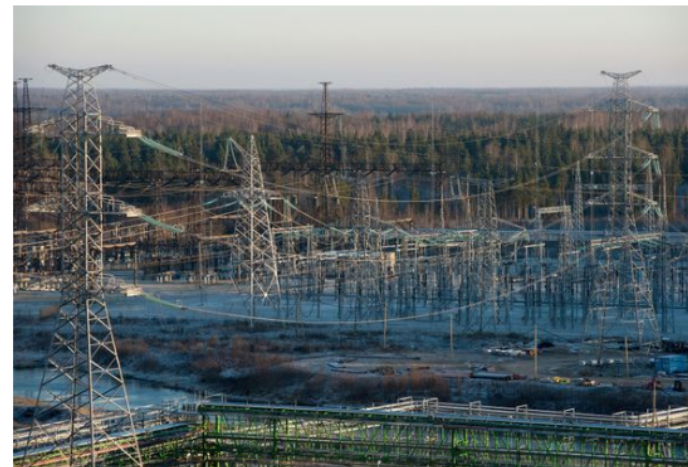
High voltage electricity power lines hang from pylons at Eesti Energia AS's Enefit 280 oil shale processing plant and energy production facility in Narva, Estonia. Photographer: Peter Kollanyi
